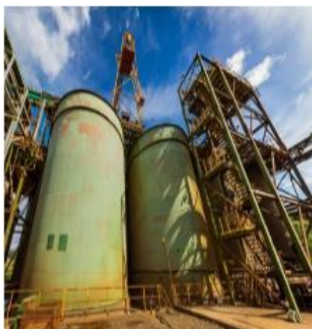
Figure 78: Pre-Leach Thickener and Conditioning Source: Amapá Minerals, 2026
